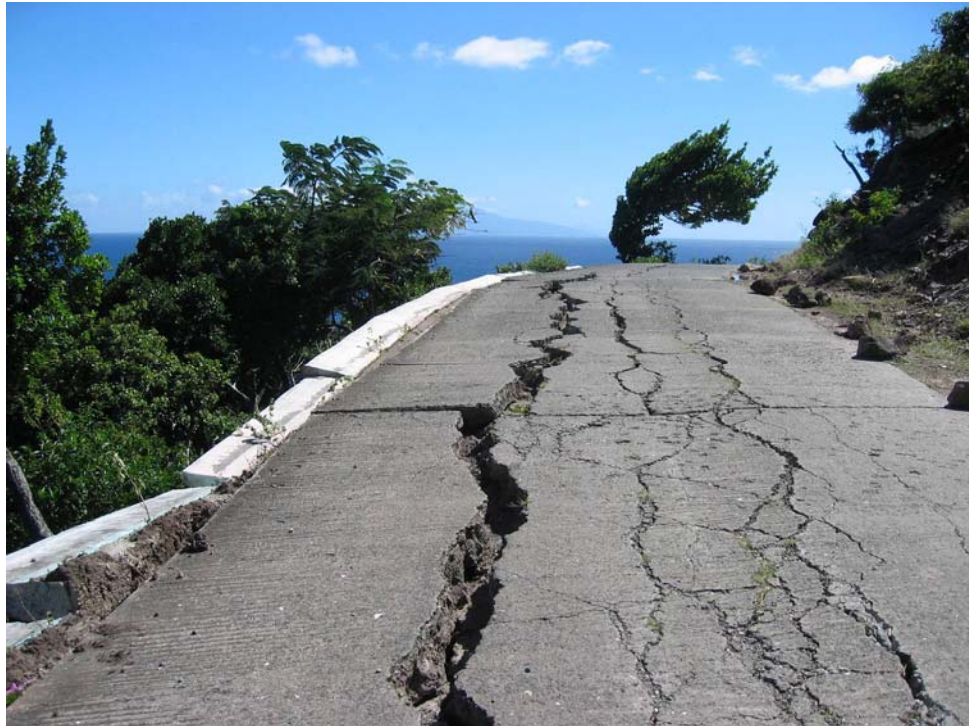
Figure 106 - RD 213 : fissurations de la route.
