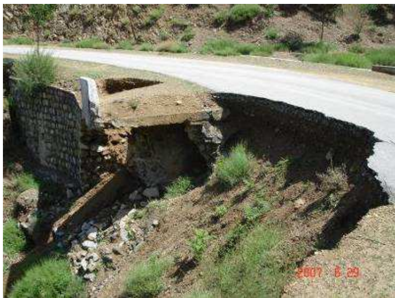
Structural damage due to a badly designed culvert on Barawal-Gal road, km 2.9
