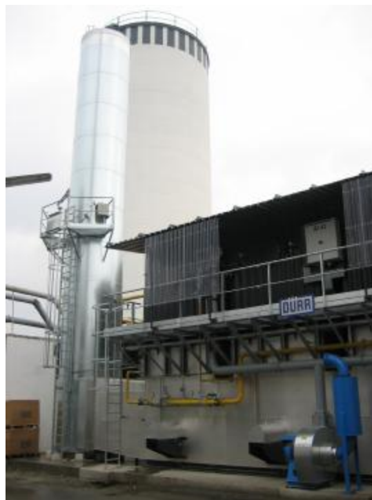
Ecopure ® RTO-Anlage at Interlübke in Rheda-Wiedenbrück, Germany.
