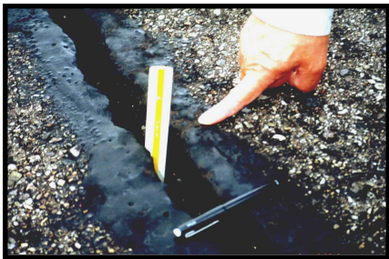
High severity cracking on the runway at Michael AAF
