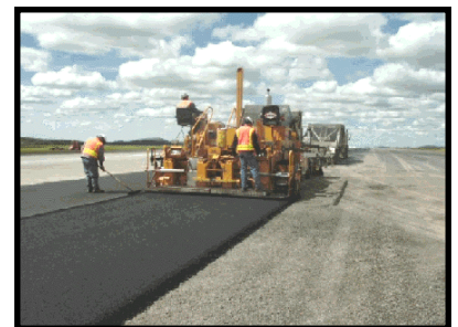
Construction of the Runway at Fairchild AFB after successfully laying pavement in a test section.
