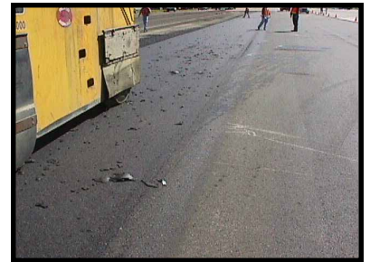
Test section at Fairchild AFB. The asphalt pavement is lifting off of the surface. USACE recommended additional rollers to keep up with the paving operation so the mix did not have time to cool.
