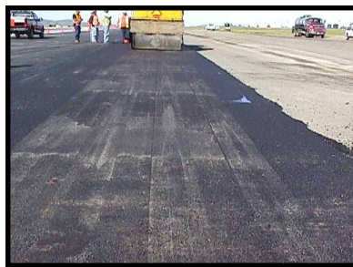
Most likely roller stopped during laydown on the test section. USACE recommended that contractor keep the rollers moving on the pavement.
