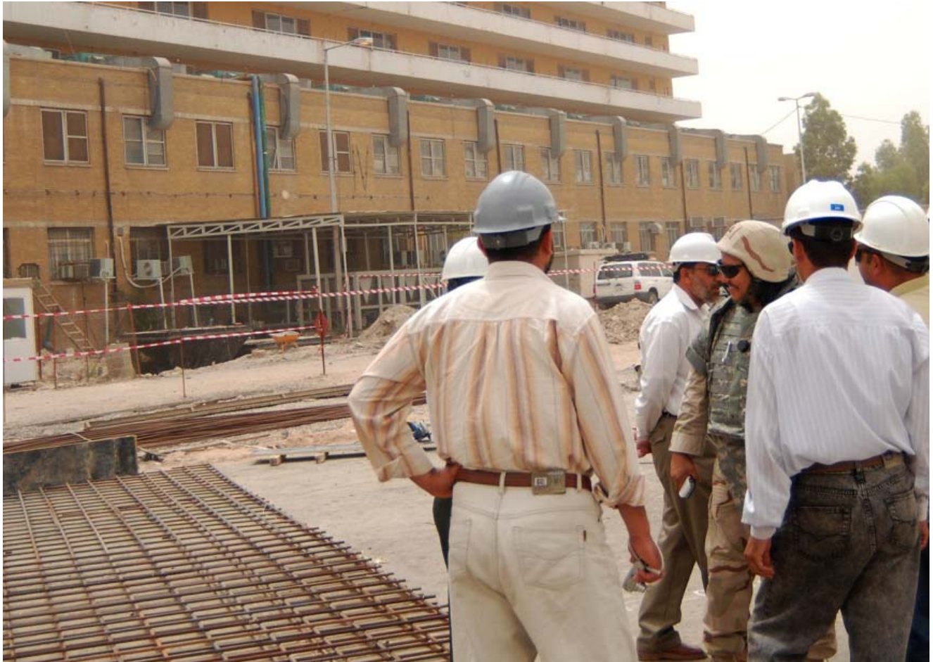
Al-Sadr hospital: (in the center) Ferdinand Guese, USACE project engineer, discusses construction with the Iraqi engineers at Al Sadr Teaching Hospital. (USACE photo by A. Al Bahrani).
