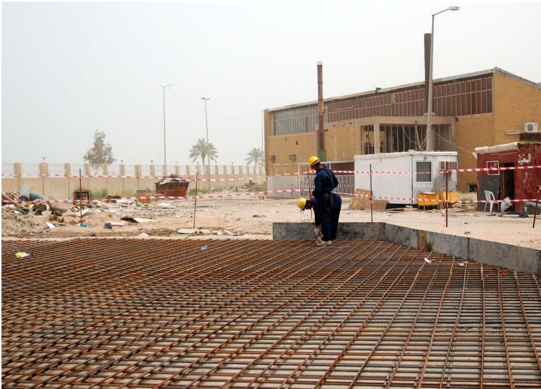
Al-Sadr hospital: Workers tie steel before placing the concrete foundation for the new 40 cubic meter waste water plant. (USACE photo by A. Al Bahrani).
