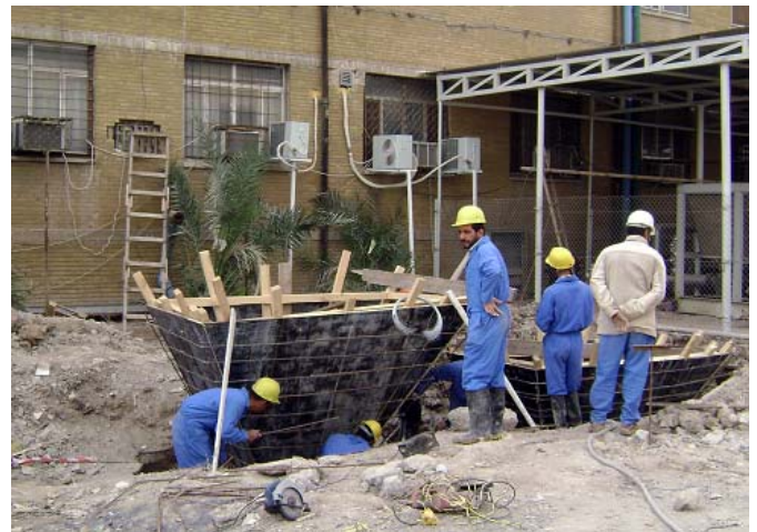
Al-Sadr hospital: Iraqi workers install wooden forms and reinforcing bar for the construction of the two new manholes. (USACE photo by A. Al Bahrani).
