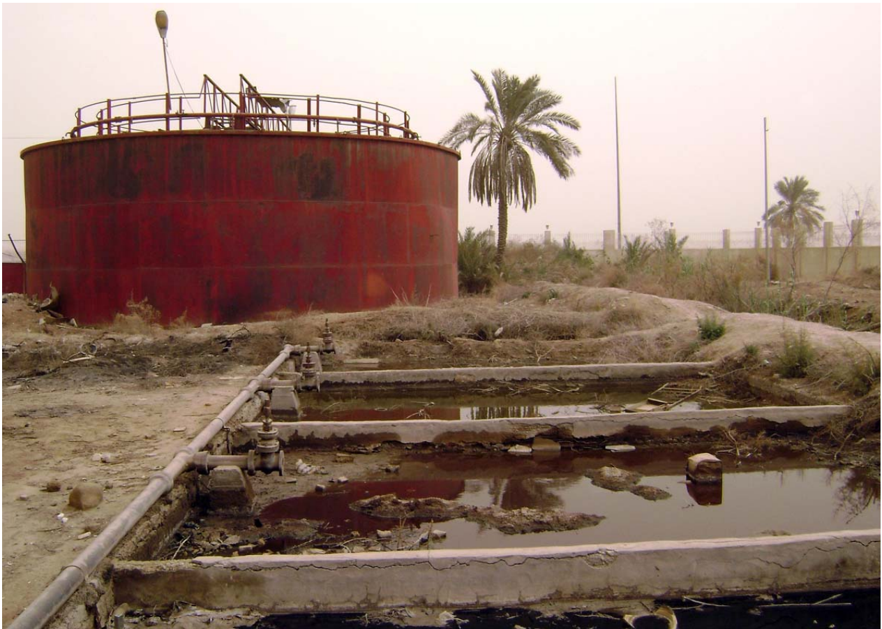
Al-Sadr hospital: The old waste water treatment plant sits in disrepair, nonfunctional for more than 15 years. (USACE photo by A. Al Bahrani).
