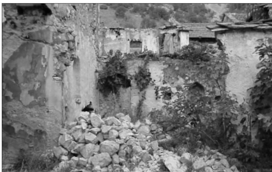
The Mahmut}ehaji} family housing complex (late 16 th and early 17 th century) in the urban complex of Uzinovi}i after its destruction (July 1993)
