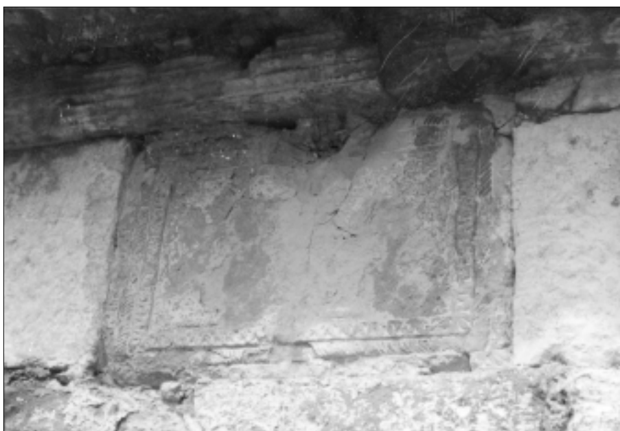
Inscription above the gate of the Mahmut}ehaji} family housing complex Damaged in 1993
