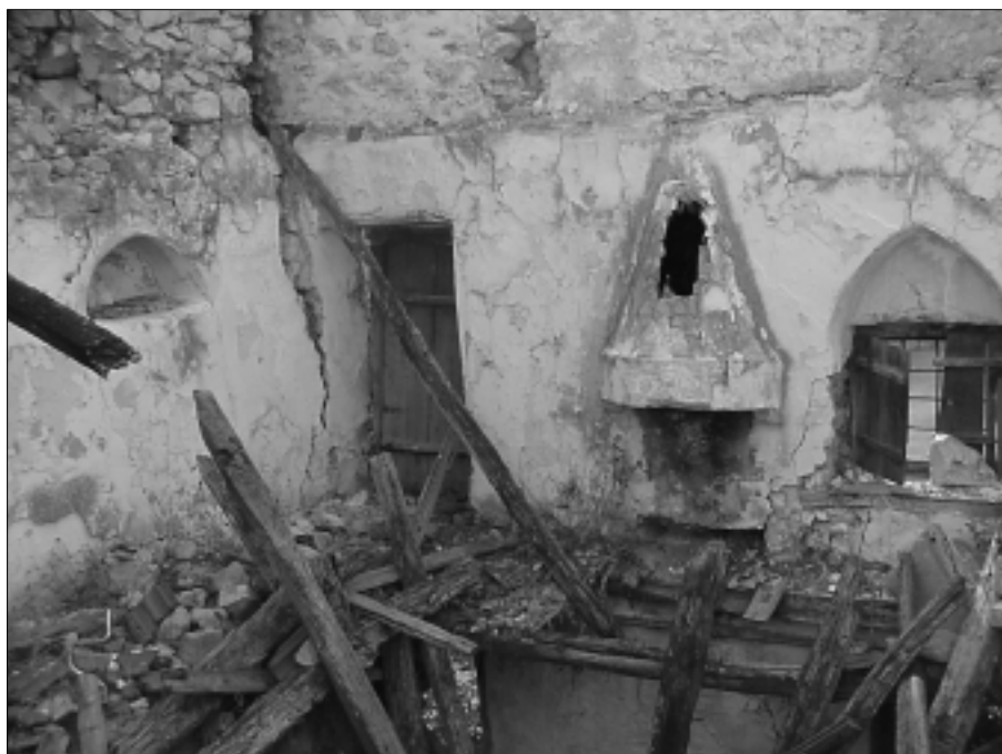
Interior of the Sarajli} family house after its destruction (July 1993)
