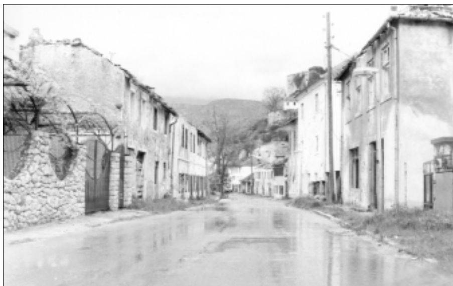
Part of the Podgrad urban complex, after many of its houses were burned out in 1993
