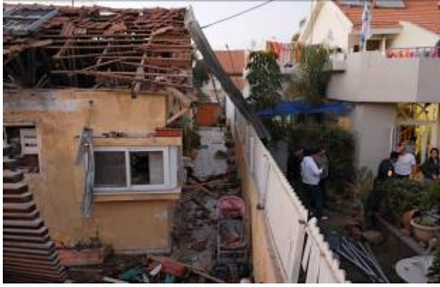
House in Sderot damaged by rocket fire (Amir Cohen for Reuters, December 13, 2007).
