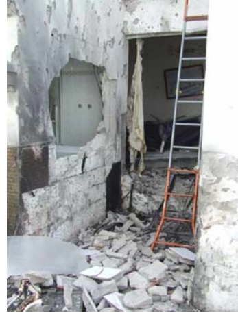
House in Sderot destroyed by direct rocket hit (Photo courtesy of the Sderot security headquarters, May 16, 2007).
