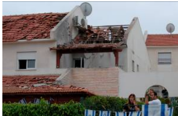
Damage done to a house in Sderot by a direct Hamas rocket hit (Amir Cohen for Reuters, May 15, 2007).
