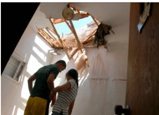
Inspecting the damage done by a direct rocket hit (Amir Cohen for Reuters, August 28, 2007).
