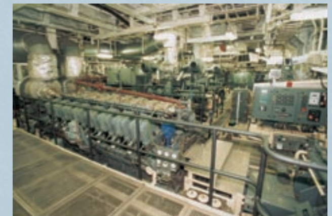
Aft Engine Room
