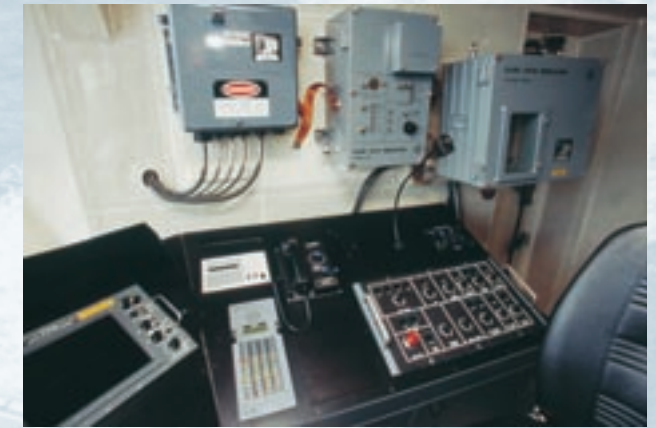
Heli Control Room
