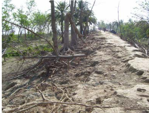
Photo 3.14. Embankment was severely damaged and this picture was taken after some initial repair of the embankment
