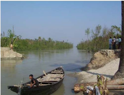
Photo 3.21. Damaged embankment due to SIDR
