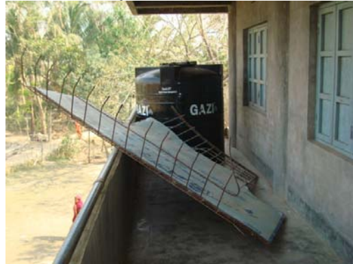
Photo 3.4. Damage gates of the cyclone shelter caused by cyclone SIDR
