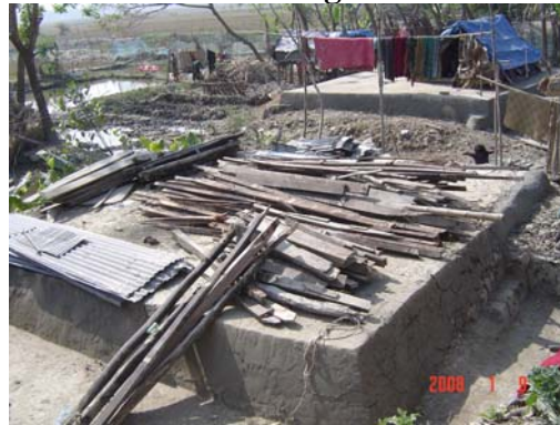
Photo 3.22. SIDR completely destroyed houses near coastal embankment
