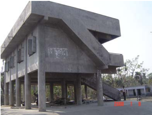
Photo 3.7. Cyclone center where severe storm surge occurred
