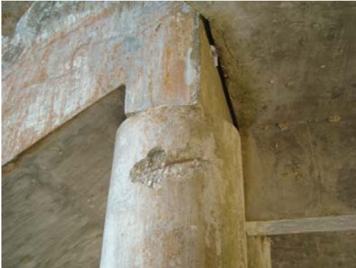
Photo 3.3. Some structural damages due to lack of operation and maintenance
