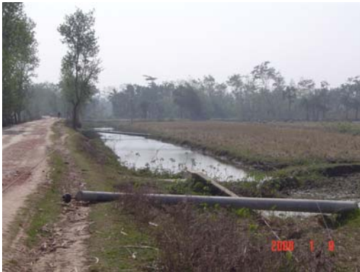
Photo 3.29. Rural electricity supply lines are heavily disrupted and fallen from cyclone
