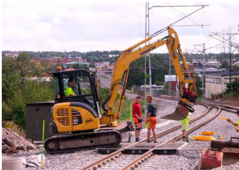
The Roslagen suburban railway has been successively renovated over a number of years. In the summer of 2007, a total refurbishment was carried out on the Rydbo-Österskär section. Starting in 2009, the Roslagen suburban railway will be fully converted to double track.
