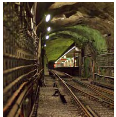
Intelligent fire alarms are being successively installed in the underground's tunnels. These alarms can tell the difference between diesel gas and foreign gas, and are also able to track the source of gas emissions.
