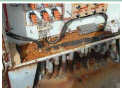
Electrical panel at Clarence Fahnestock State Park
