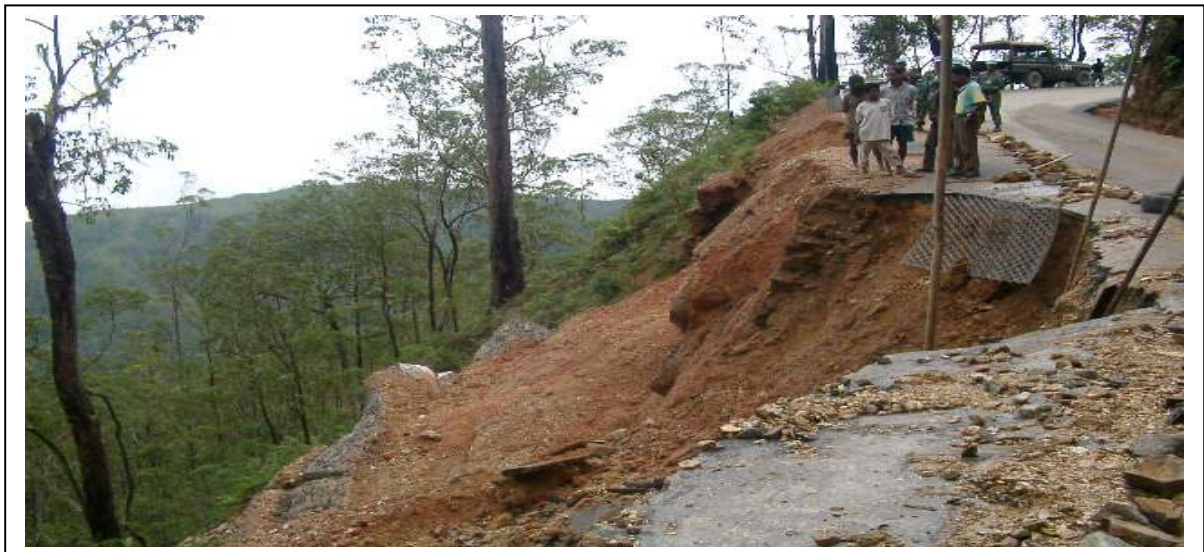
Photo 3: Landslide on the Dili-Aileu-Cassa road
