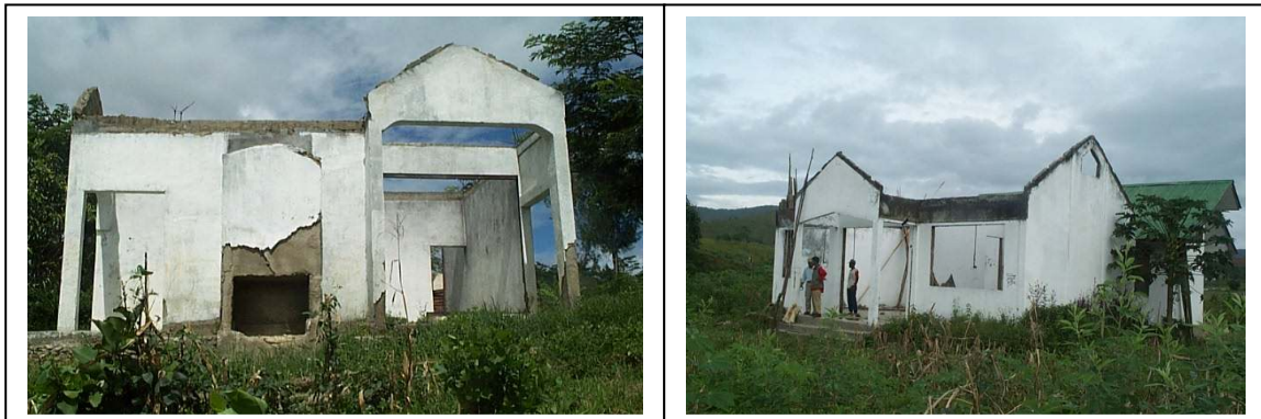
Photo 4: Government Buildings Awaiting Rehabilitation
