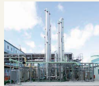
Biogas Upgrading System
