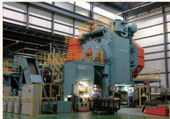
Four 6,300-ton mechanical presses have been installed to enable KAAP to respond to an expected increase in demand.
