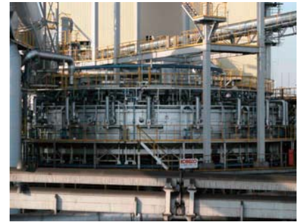
A FASTMET® plant at Nippon Steel Corporation's Hirohata Works
