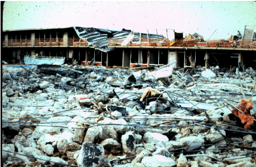
Destruction at the Best Western Bossier Inn. View from the ground. (Photo courtesy of Ernest Ethridge)
