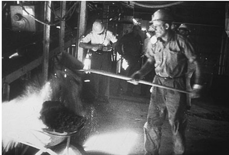
Workers cleaning up generate more asbestos dust
