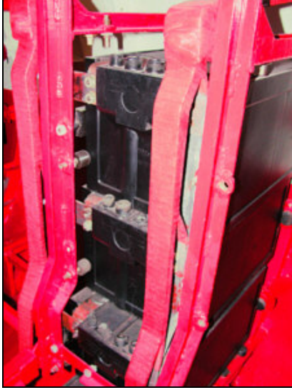
Figure 35: Preserved battery stack in the aft battery room of midget Ha-14 .
