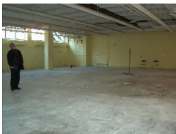
Before (taken in early May 2005 – with Vladimir Baranov inspecting the duct work)
