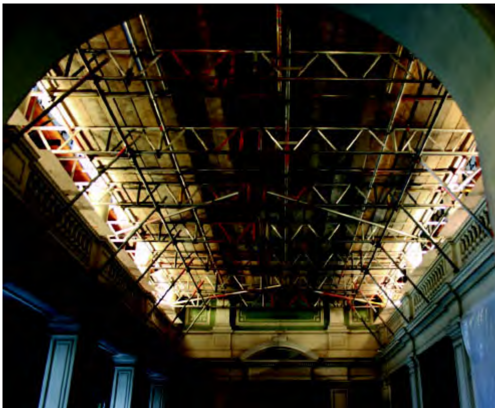
The Library Reading Room with the scaffolding and boarded false ceiling to allow the day-to-day work of the Society to continue beneath it.
