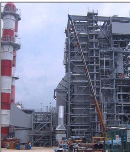
SUCCESSFUL MECHANICAL COMPLETION 400 TPH GAS AND OIL FIRED BOILER, SEMBCORP, JURONG ISLAND SINGAPORE
