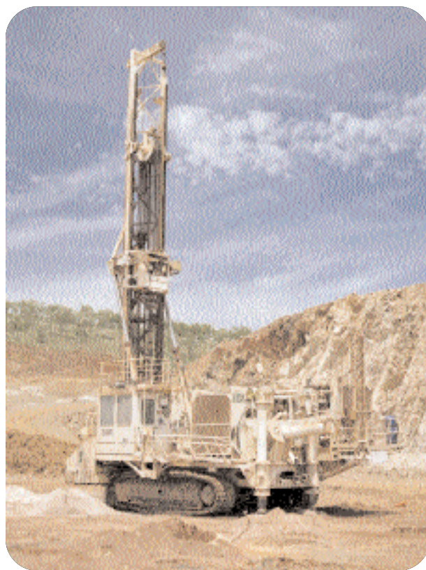
Figure 8. Mobile drill rigs at Argyle make holes for the explosives needed to mine the ore.
