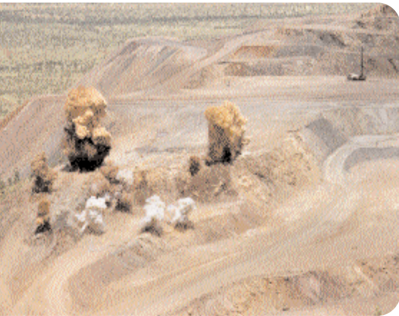
Figure 9. At Argyle, explosives are used to break up the lamproite ore and its overburden, so that it can be removed more easily.
