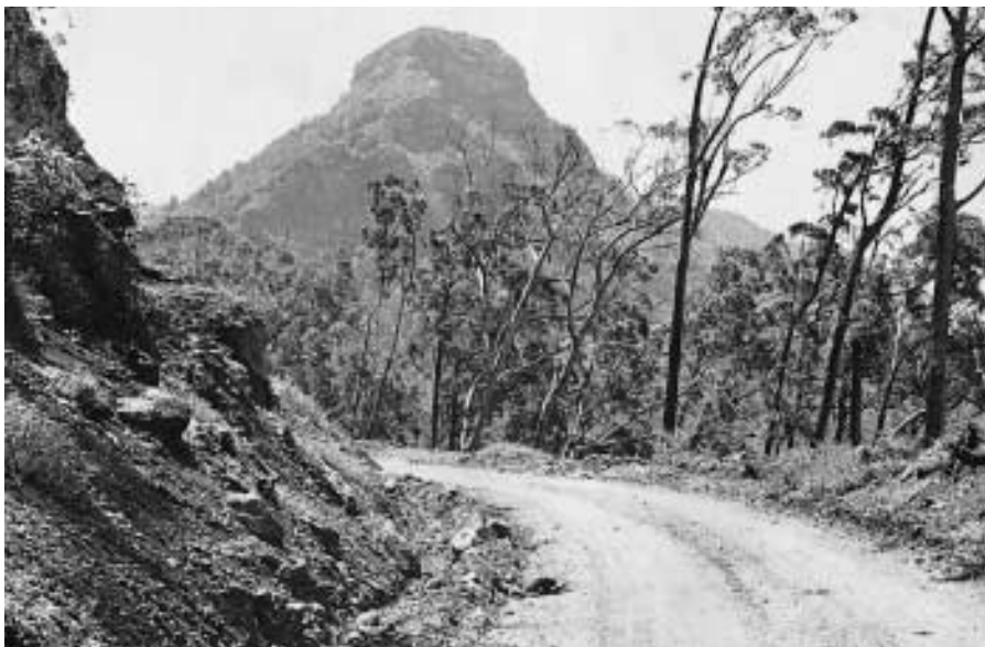
Road building projects, such as those at Cunningham's Gap, provided unemployment relief during the Depression.
