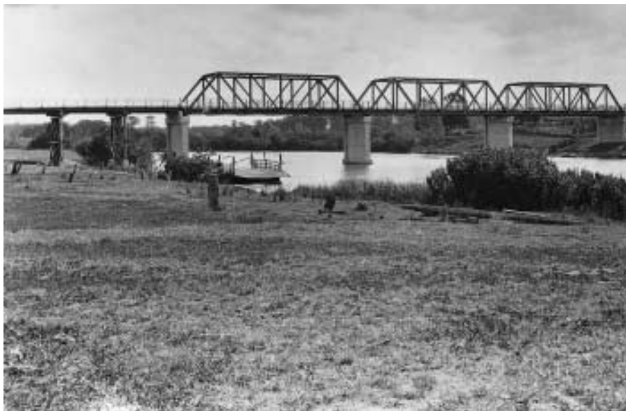
The Logan Toll Bridge, 1934. Tolls were introduced to meet some of the difficulties of finance.
