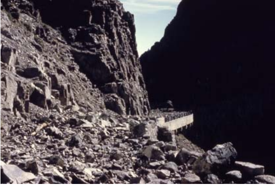
Rock fall on Golden Gate Road, Yellowstone National Park following August 17, 1959 Hebgen Lake Earthquake
