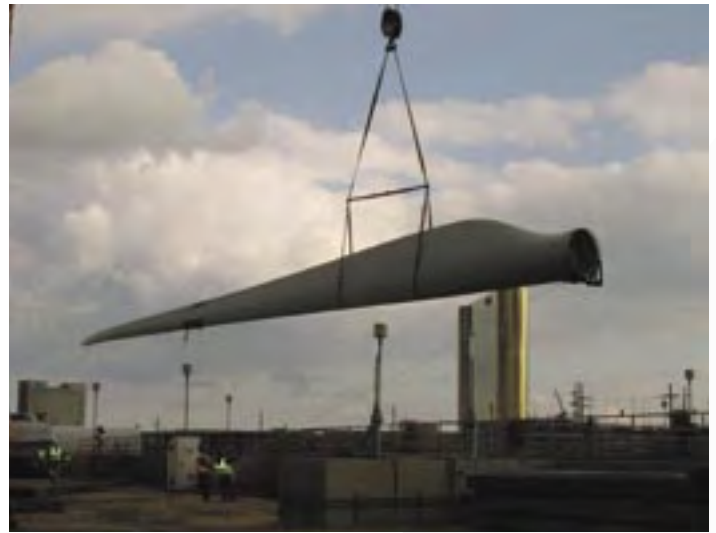
During the construction of the Jersey-Atlantic Wind Farm a 120 foot long windmill blade is hoisted into the air.
