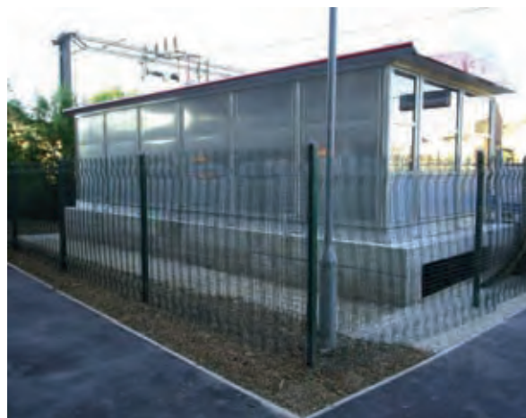
Runcorn – recent NSIP upgrade
