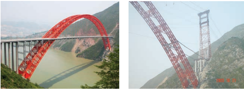
(a) Finished (b) Under construction Figure 12: Wushan Yangtze River Bridge in Chongqing
