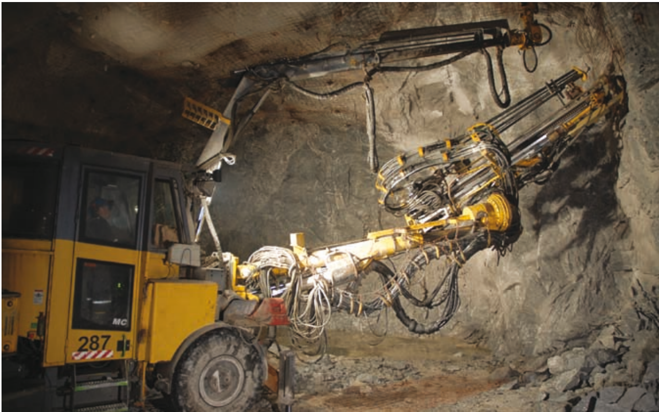
Underground at Diavik a bolter operator attaches screen in one of the tunnels.
