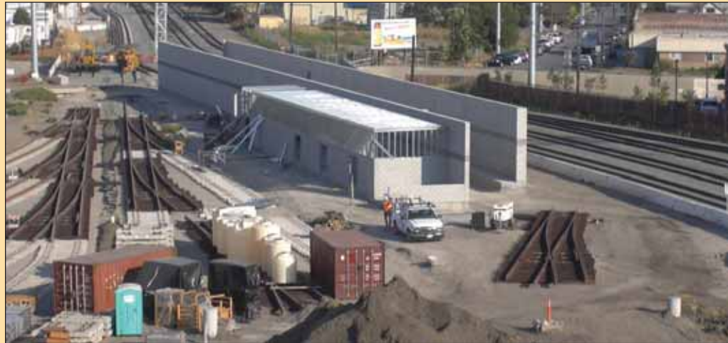
North of the maintenance shop, a train-sized version of a carwash is under construction. The trainwasher and water treatment plant buildings have been constructed and are ready for the equipment to be installed this fall. Each day, trains will be driven through it so they receive a washing and scrubbing that they now only get twice a year.
