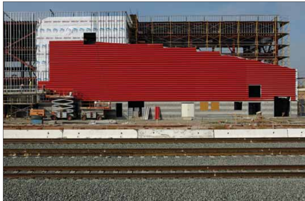
Long panels of red corrugated steel add to the aesthetic look of CEMOF's three-story maintenance shop, which is rising next to the Caltrain tracks. The site is bounded by Coleman, Lenzen and Stockton avenues and by West Taylor Street on the north.
