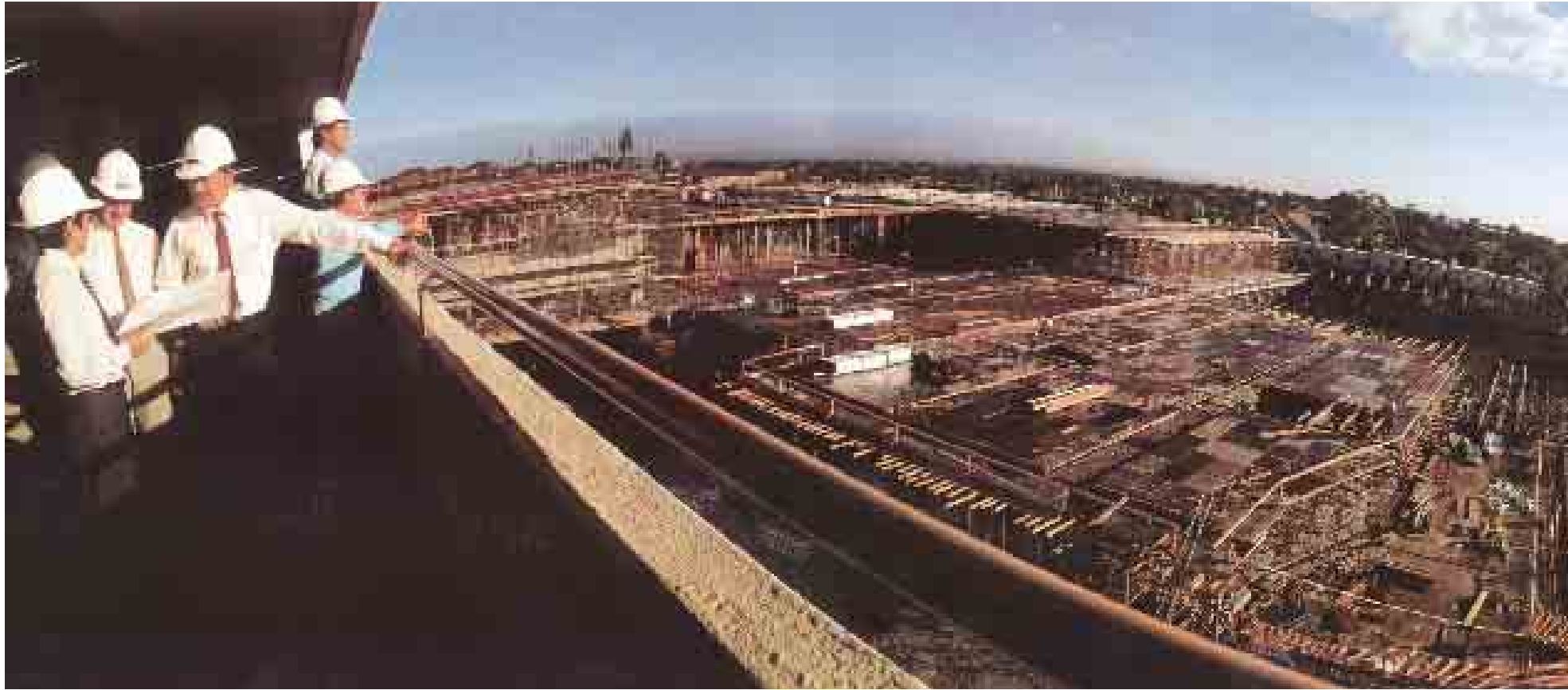
The redevelopment of Hurstville in Sydney (1988–1990) more than doubled the size of the centre.
