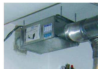
Central exhaust ventilator in the cellar, adapted to the air chimney
