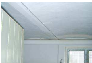
Airtight plastering in good condition under a T-beam arch brick cellar ceiling
