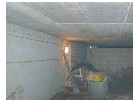
Concrete cellar ceiling without insulation. High U-value = 2.2 W/m 2 . 10 cm insulation from below can reduce heat losses by 85 %
