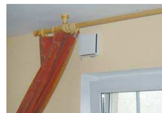
Fresh air inlet valve beside a window
