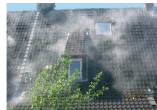
Smoke pressed out by a Blower Door fan to show the roof leaks
