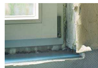
Foam-filling of the new window installation gap is not sufficient. The connection between window frame and wall must be airtight and vapour-retarding all around.
