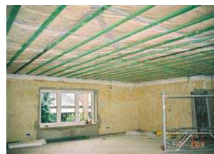
New air- and vapour-tight foil installed from below with foil connections to the walls
