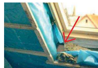
Missing connection between roof window frame and airtight foil
