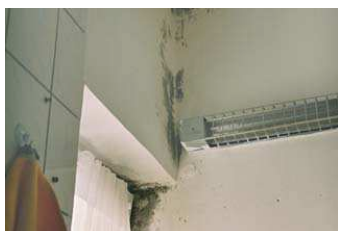
Mould in the corners of a bathroom caused by a geometrical thermal bridge to the cold outside
