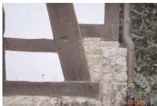
Cracks and gaps are often not visible
