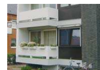
Thermal bridges caused by concrete components (wall / balcony)
