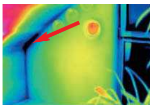
Cold room corner caused by untight connections between walls and roof
