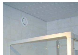
Exhaust valve for used air in a bathroom
