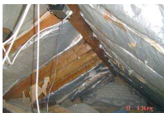
Defective aluminium-coated roof insulation and airtight layer
