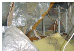
Damaged and not repaired airtight foil in a roof causes high heat losses
