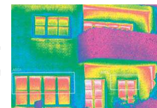
Thermography shows the higher surface temperatures near thermal bridges
