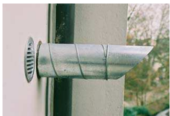
Fresh air supply is now from the garden side
