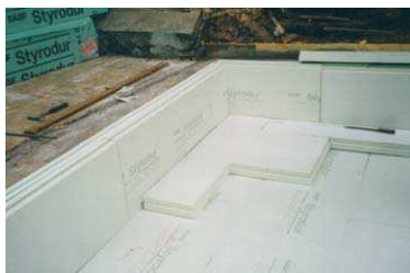
Two-layered insulation with Styrodur 5000 floor boards within the ring footing for the natural stone walls
