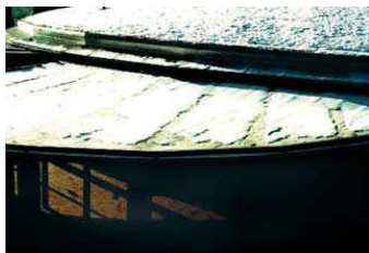
Thermal bridge caused by wooden rafters without insulation above or below
