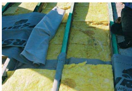
Pitched roof with plastering inside. A mineral wool layer of 3 cm has already been installed as foil protection. Additional insulation is being prepared. Additional upper laths are also visible.
