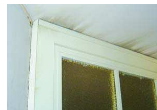
Untight hall door to staircase
