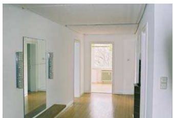
Fresh air pipes under textile-covered corridor ceilings
