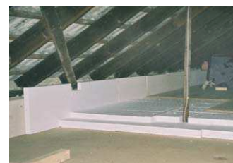
Reducing the thermal bridge of a concrete beam in a cold loft by 10 cm flanking insulation
