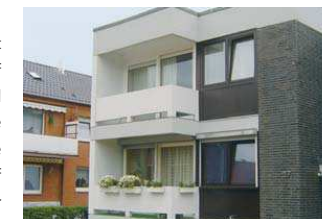
House of the early 1970s with many thermal bridges caused by concrete elements
