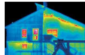
Heat losses through an air-leaky connection between front wall and roof
