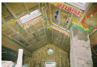
Roof insulation from inside with two additional insulation layers and a diffusion-variable membrane
