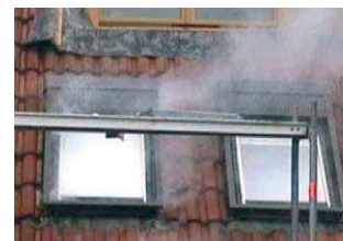
Untight roof window frame - made visible with artificial smoke
