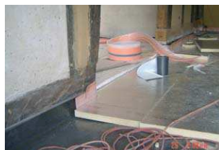
Lowered sole plate, newly waterproofed with 6 cm PU insulation on top (0.025 W/mK)
