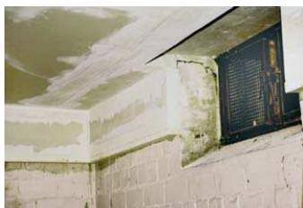
Reduced thermal bridges on a cellar ceiling by extending the insulation (6 cm thick) to the upper part of the walls (50 cm)
