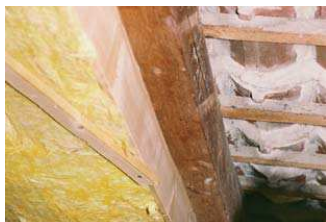
A shelf fixed laterally to the rafters provides additional space for 24 cm insulation.
