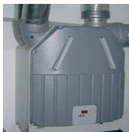
Ventilation system with 90 % heat recovery accommodated in the toilet
