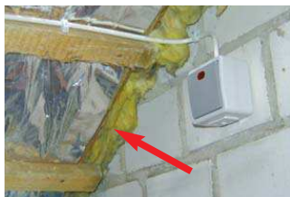
Airtight foil not connected with the wall. A 5 cm wide strip around the roof is untight.
