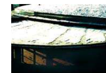
Thermal bridges caused by wooden rafters
