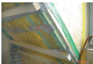
Two layers of laths inside the rafters provide more space for insulation.
