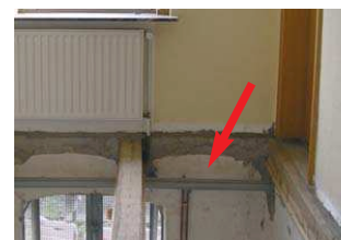
Inner plastering of the outer wall is missing on wooden ceiling level (here opened)
