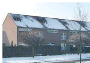
Irregularly melting snow on a roof is an indicator of air leakage or thermal bridge
