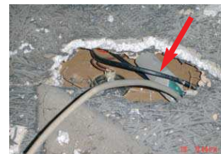
Holes in a loft ceiling not closed after installing a recessed luminaire
