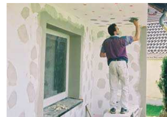
Reducing the thermal bridge of a concrete balcony by applying 6-8 cm insulation on both sides
