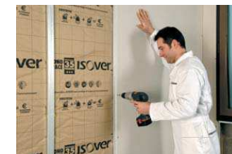
Internal insulation of an outer wall with resilient bars and gypsum boards
