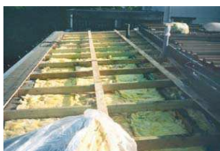
Flat cold roof opened from the top with additional joists to provide space for a total insulation layer of 24 cm thickness
