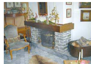
Open fireplace drawing fresh air from the room. It causes high ventilation heat losses regardless whether a fire is burning or not.
