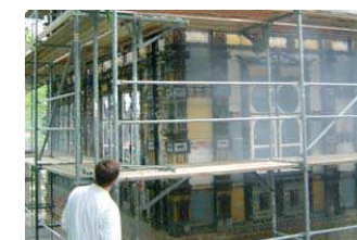
The outgoing smoke shows air leaks on a historical facade
