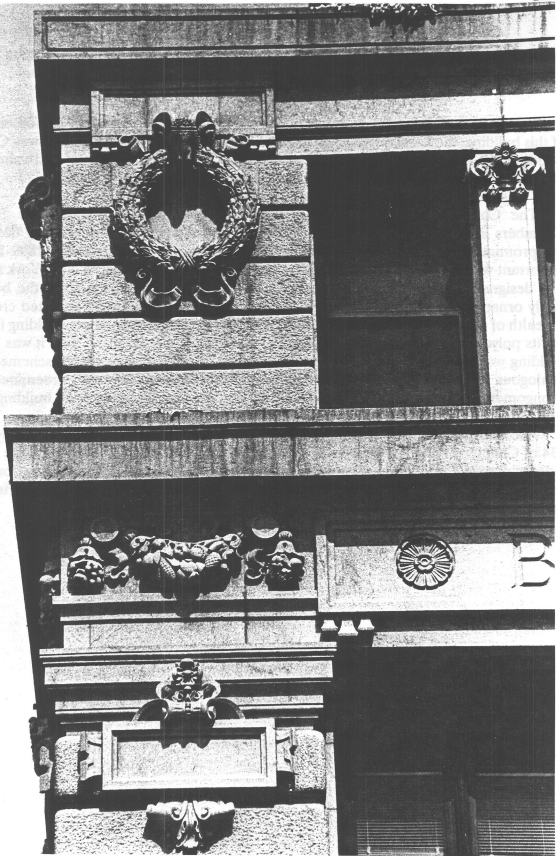
Fig. 2: Detail of ornament at second and third story, Broadway Facade. (Photo Credit: Carl Forster.)
