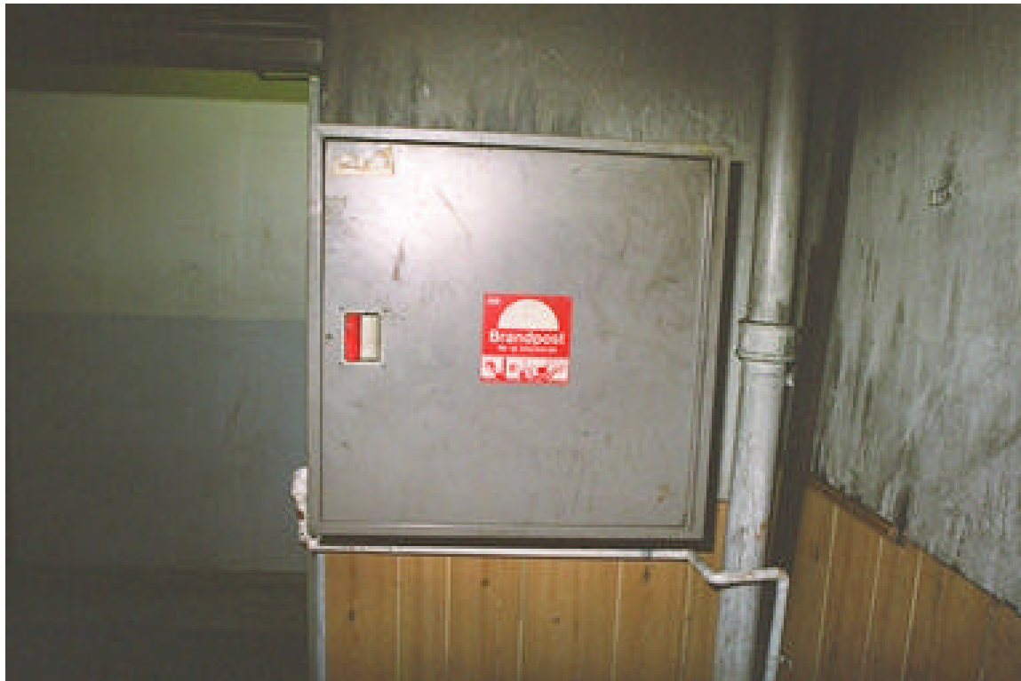
Photo No. 1 – An occupant-use hose cabinet was located in the entrance corridor adjacent to the exit stairway. (NFPA)
