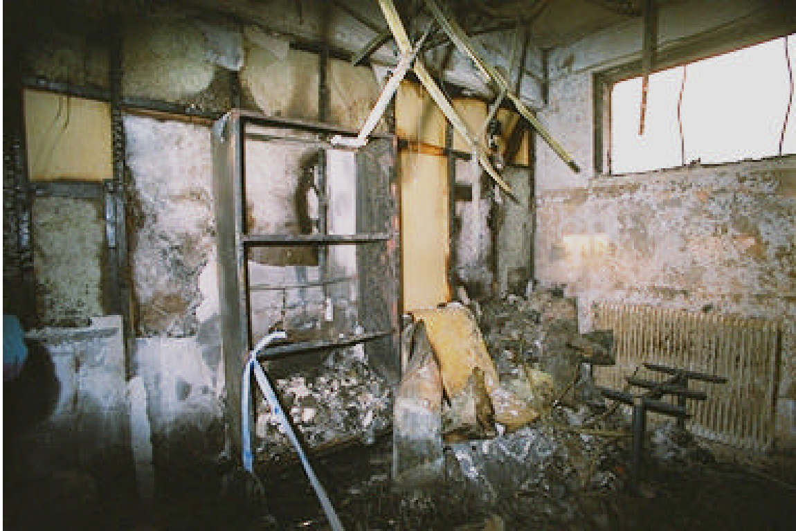
Photo No. 11 – This is the wall that separated Room #203 from the main hall. At the top of the wall were glass panels that failed during the fire, allowing smoke to spread into this room.
