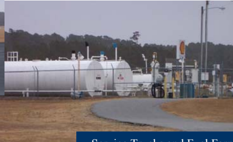
Service Trucks and Fuel Farm
