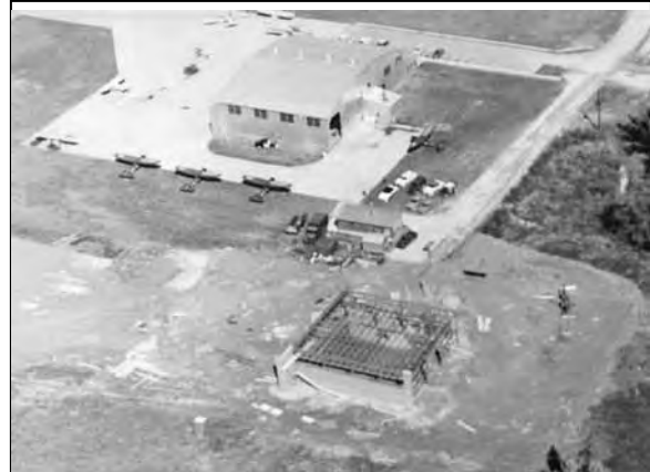
1958 photo of construction underway for the Army Aviation Maintenance Shop at Capital City Airport. The hangar is still in use today by the Division of Air Transport. Four I-19s are shown around the hangar.
