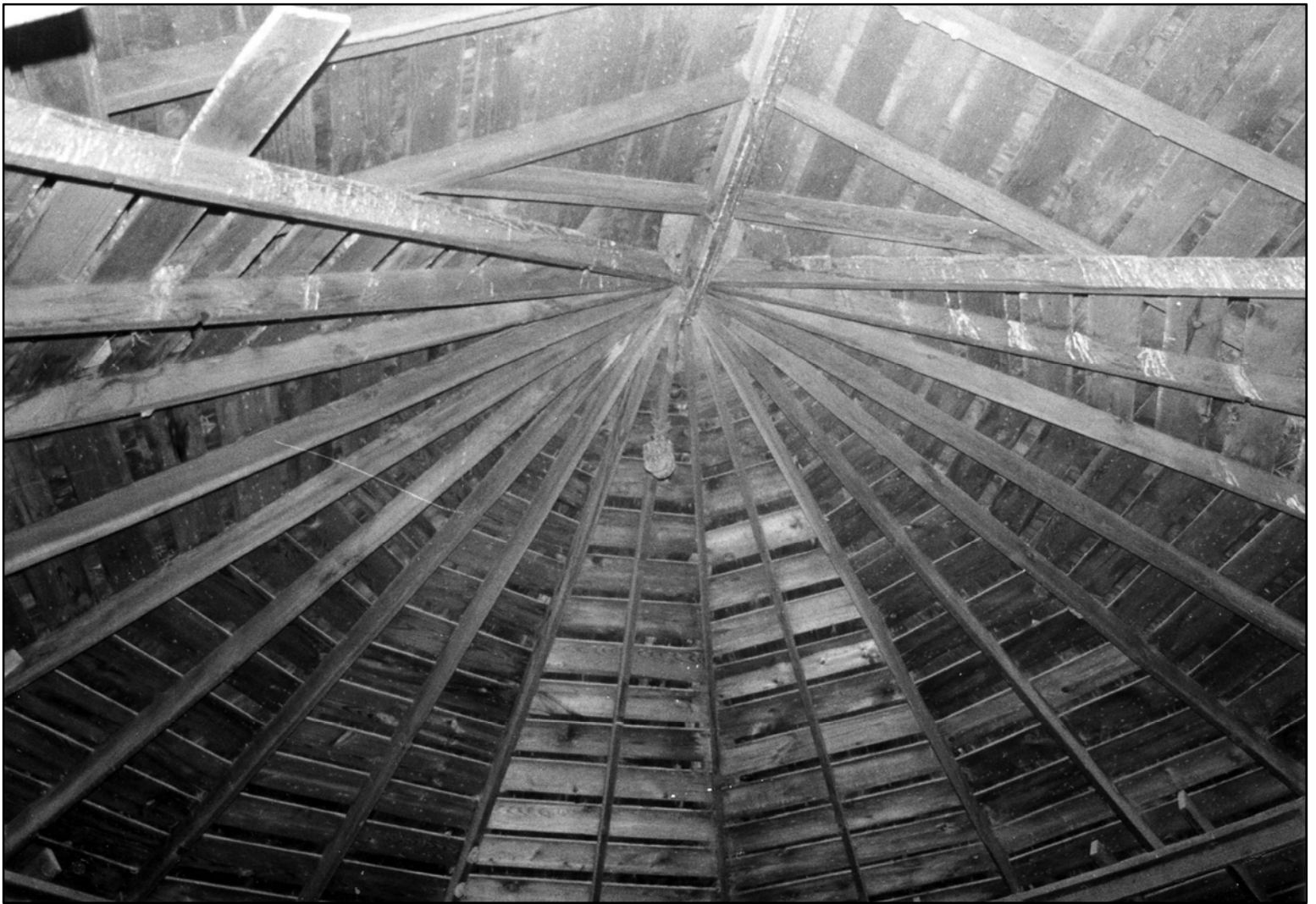
Photo 6 of 6 – interior view looking up showing roof truss system Photo by Janet Jeffries Spencer, May 1985, NSHS (8505/3:24)
