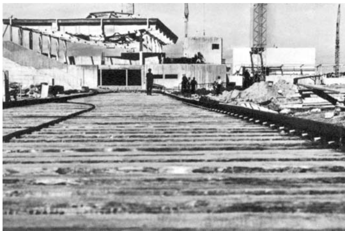
Construction progress in Kiel: Pile foundation at the sandy shore area of the Kiel inlet; the terrace has been com- pleted, the rough construction of the swimming hall — in the background, with the pool — is almost finished; unbroken progress of the rough construction on the main tract running from north to south with the boat house and swimming hall in the foreground, apartment houses in the background. One year after the laying of the cornerstone all the rough construction of the buildings of the Olympic Yachting Center was finished.
