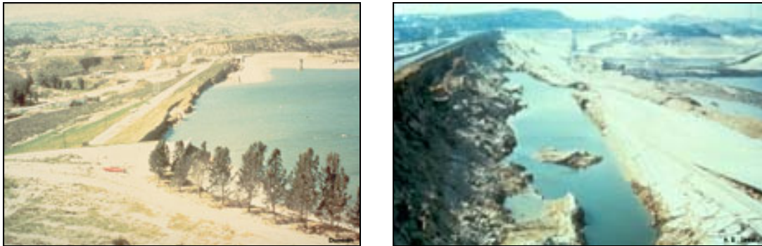
Figure 13. Aerial view of the crest (left) and the slide in the upstream shell of the Lower San Fernando Dam, in California, after the 1971 San Fernando earthquake
