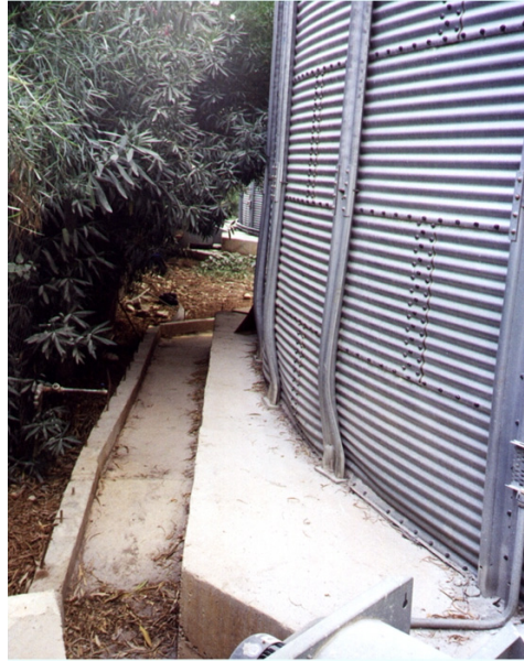
Figure 15. Damage at the OSB Amylum Factory by the 1995 Ceyhan, Turkey, earthquake
