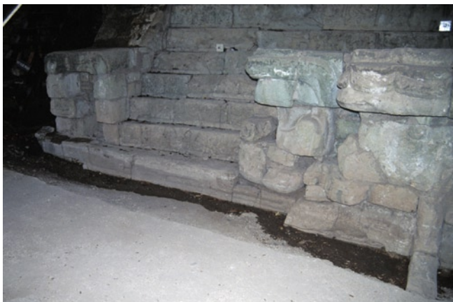
Figure 156 Accumulation of rainwater at the base of the Stairway during a heavy rainstorm.
