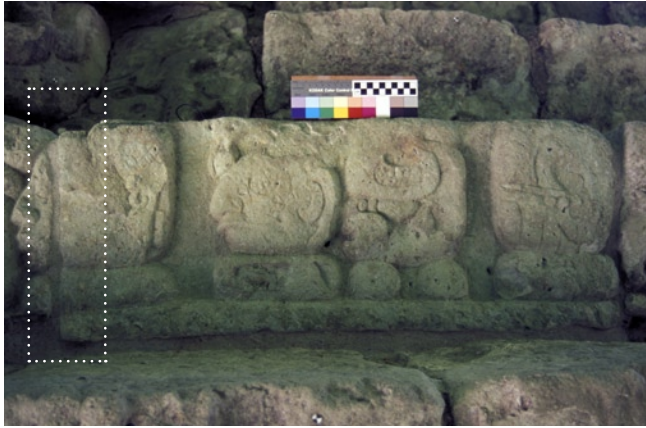
Figure 143 Block 407, step 41, after a trial treatment in which the color of the edging and fill mortar was matched to the stone surface by the addition of mineral pigments to the lime mortar (at the left).
