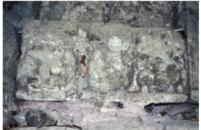
Figure 95 Block 408, step 43. Previous consolidation treatments, biological growth, and loss of repointing mortar can be seen.
