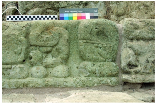
Figure 146 Repointing of treatment trial block 407, step 43 (left), and missing mortar under the adjacent block (right).
