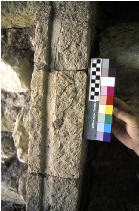
Figure 139 A crack within north balustrade blocks N38 and N39.
