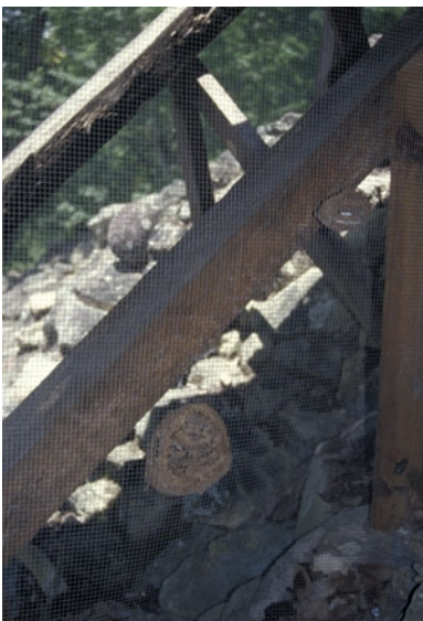
Figure 120 Metal screening leaf barrier to the north of the Stairway, with wasp's nest.
