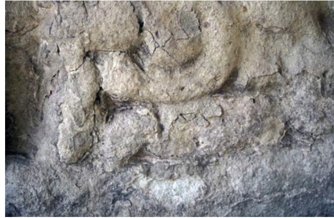
Figure 142 Block 71, step 11, with flaking and detached surfaces that require stabilization.
