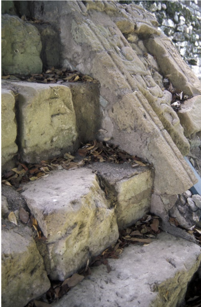
Figure 121 Accumulation of leaves on the south side of the bottom portion of the Stairway.
