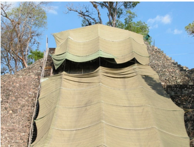
Figure 132 The shelter, which was installed in February 2001, with a tear caused by high winds in 2005, in the same location where the tarpaulin was previously repaired.
