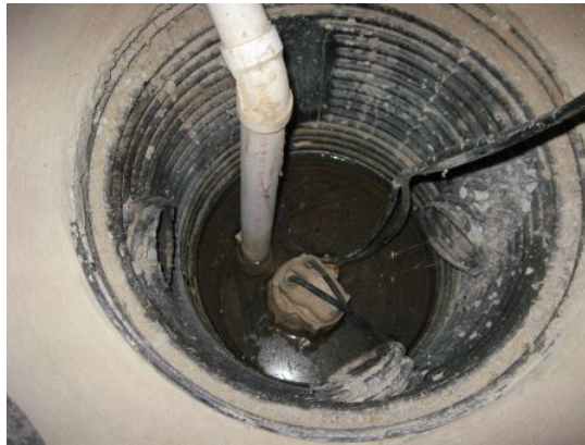
Figure 6.17: A sump crock.
