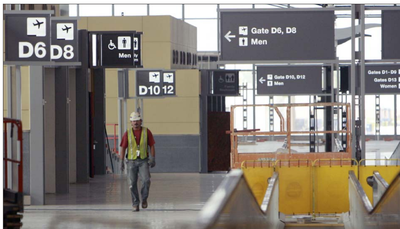
This is Concourse D, under construction in the second phase of Raleigh-Durham International's Terminal 2. The project employs 450 construction workers, making it one of the Triangle's largest public works projects.
