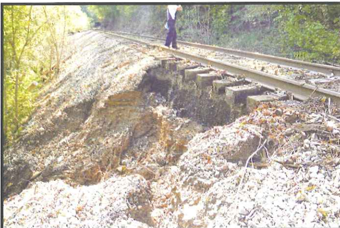
Several washouts on the Hiwassee Line required repair. This one is near Appalachia Powerhouse.
