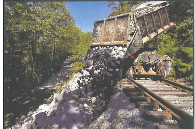
A leased hi-rail dump truck is seen placing fill near Spring Creek Road. Photos by Mike Little.
