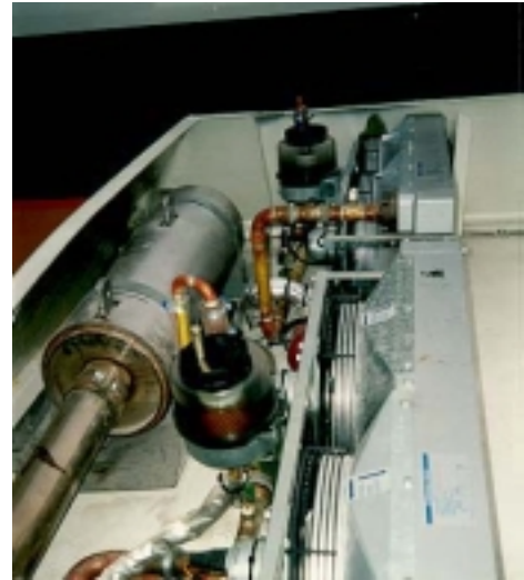
Fig. 48. The catalytic converter on the roof.
