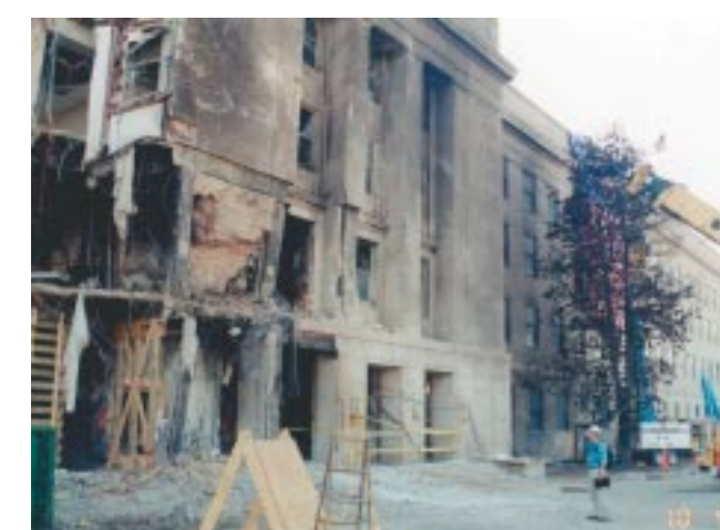
Figure 5.10 Exterior evidence of fire to the south of the impact area
