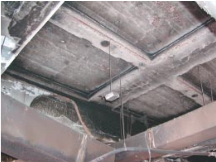
Figure 6.12 Fire damage to third-floor (light well) beams
