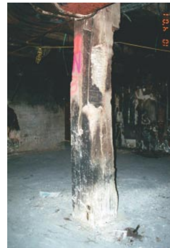
Figure 5.19 Column 3N damaged by impact and fire
