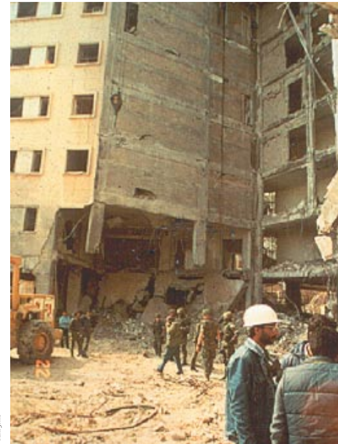
Figure 7.7 Reinforced-concrete frame with masonry filler walls acting as a vertical diaphragm to compensate for column loss
