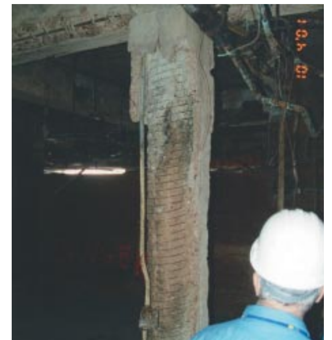
Figure 5.31 Fire damage to column in second story
