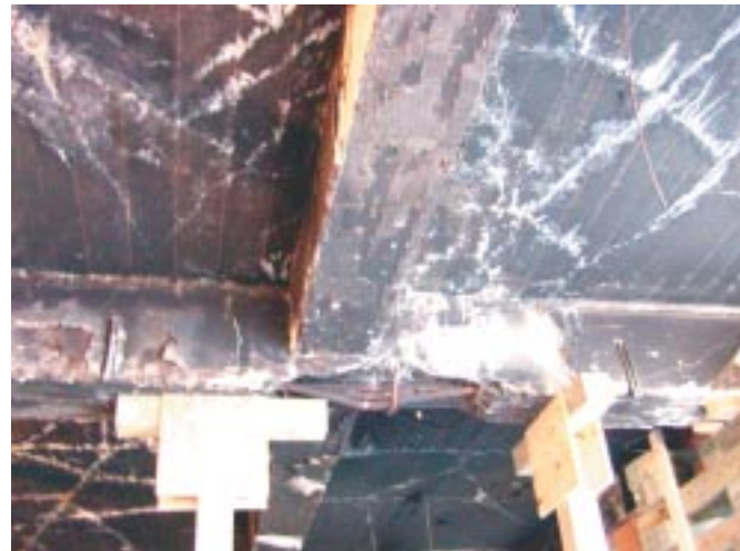
Figure 6.14 Fire-damaged second-floor beams
