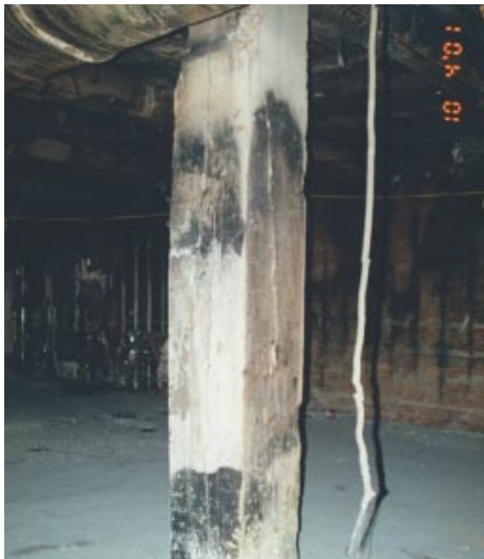
Figure 5.24 Cracked column 5N
