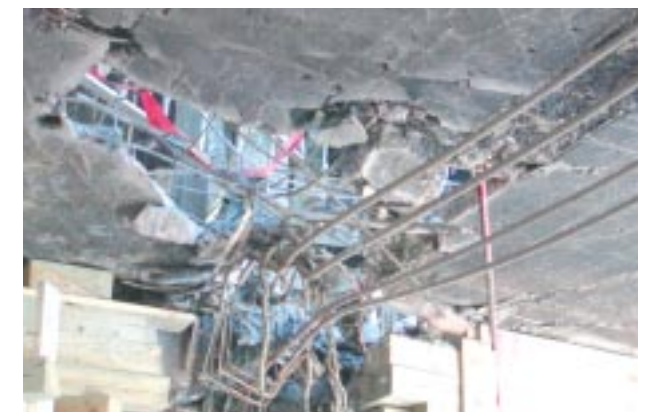
Figure 5.29 Concrete stripped from floor beam
