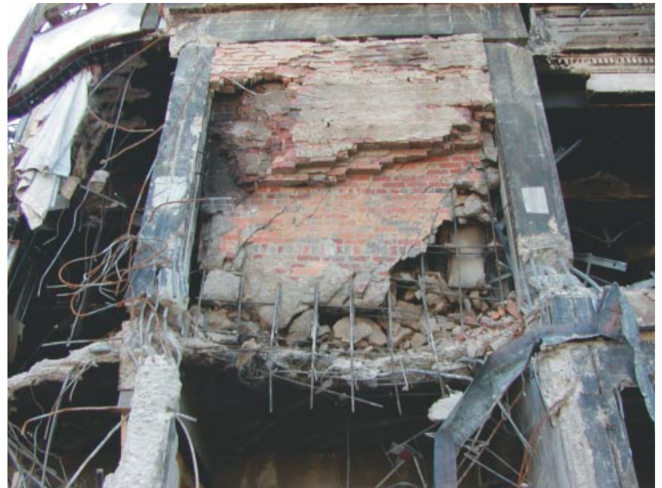
Figure 5.12 Gashes from impact of right wing
