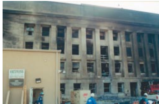
Figure 5.15 Broken conventional windows
