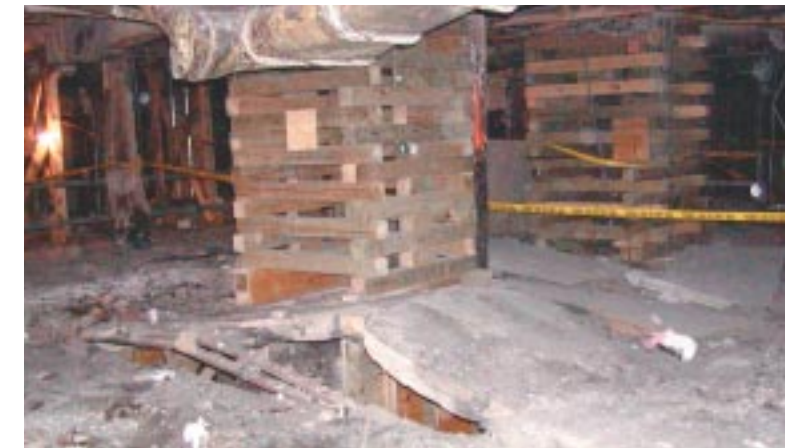
Figure 5.27 Breached second-floor slab
