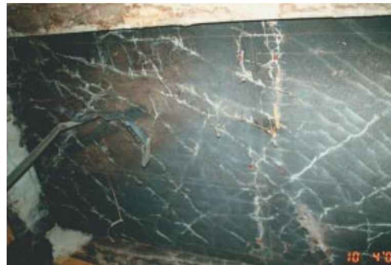
Figure 5.28 Crack patterns in second-floor slab
