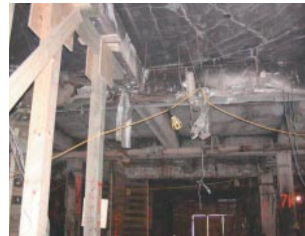
Figure 5.26 Impact damage near column 6K
