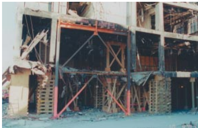
Figure 5.5 Missing first-floor columns 11A, 11B, and 11C
