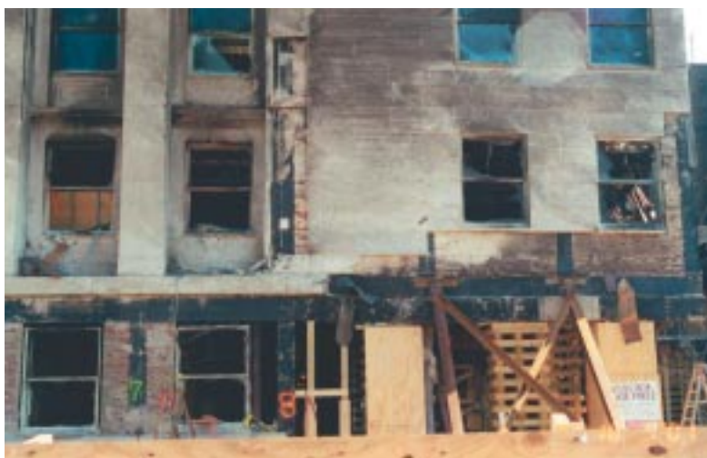
Figure 5.6 Facade damage to the north of the impact area
