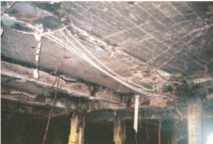
Figure 6.13 Concrete stripped from second-floor beam at grid 9 between grids A and B; extensive cracking in slab
