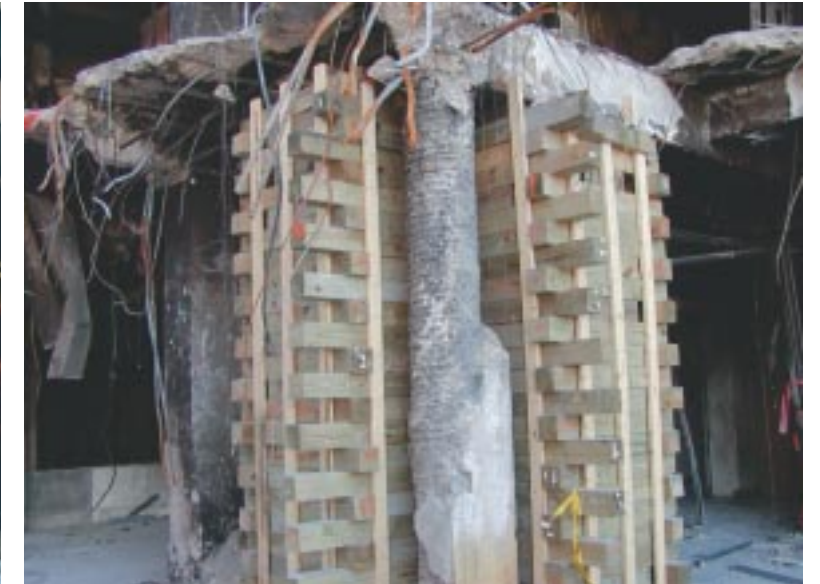
Figure 5.18 Column 15B with concrete cover removed by impact
