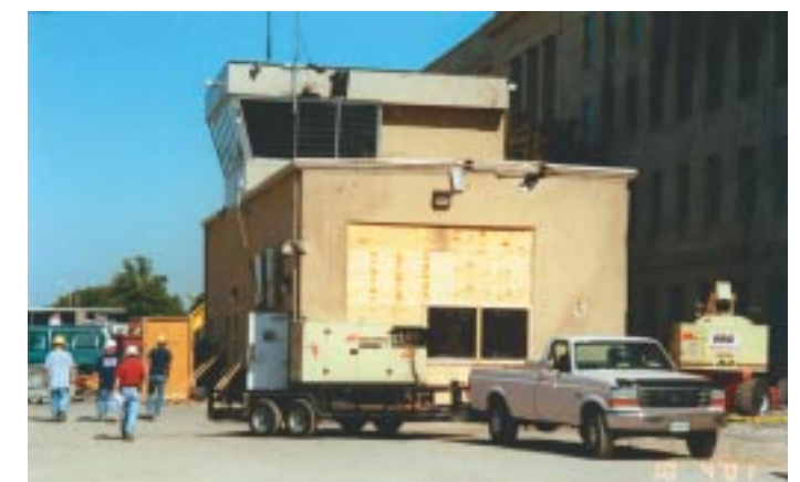
Figure 5.13 Damage to fire station
