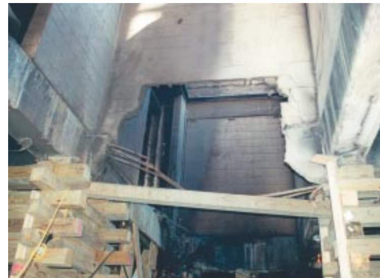
Figure 5.30 Missing beam in air shaft
