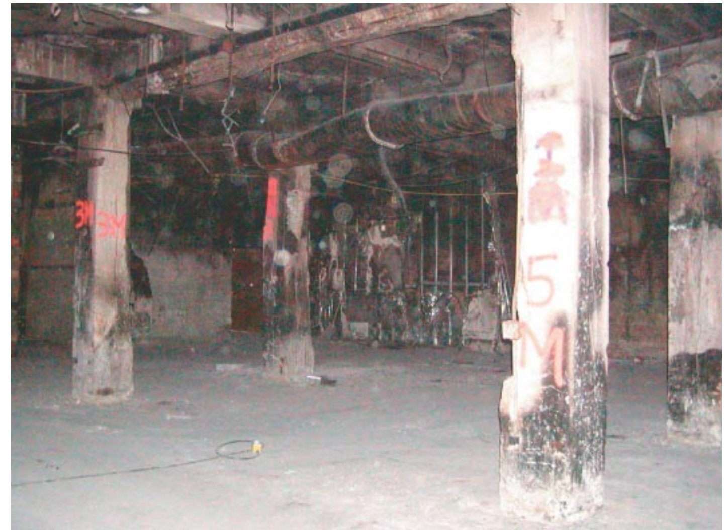
Figure 6.8 First-story columns 5N and 5M
