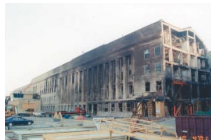
Figure 5.9 Exterior evidence of fire to the north of the impact area
