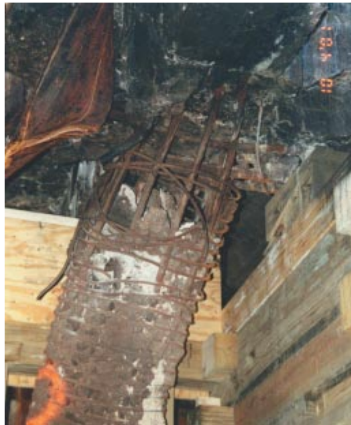
Figure 5.22 Top of column 3L, still attached to underside of second-floor framing
