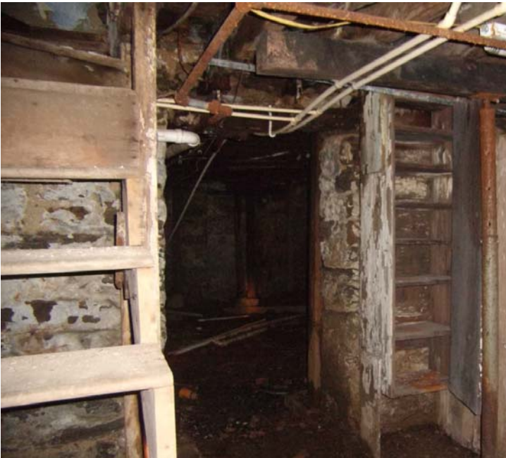
Image of opening between from the main house basement into the addition basement from October 2009
