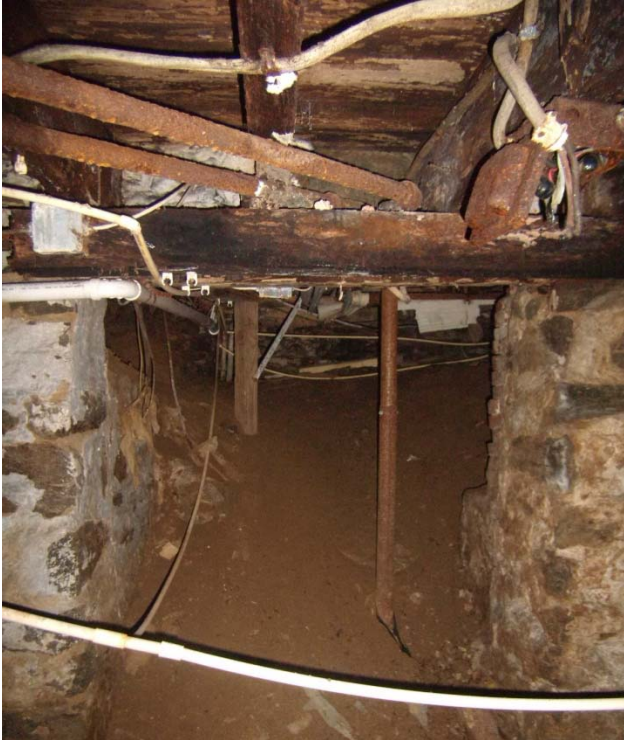
Image of the Single story addition crawl space from the two story addition from October 2009
