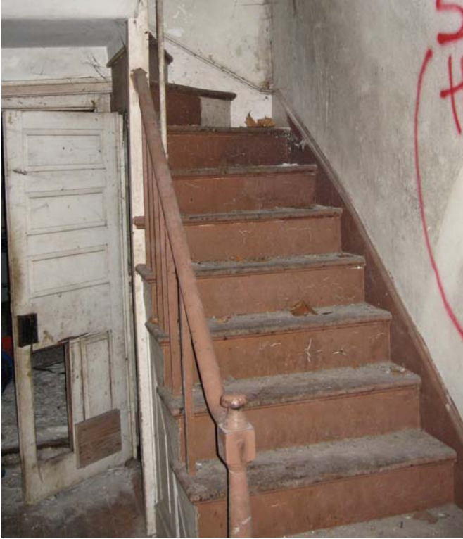
Image of the newel and rail from the main house first floor from July 2009
