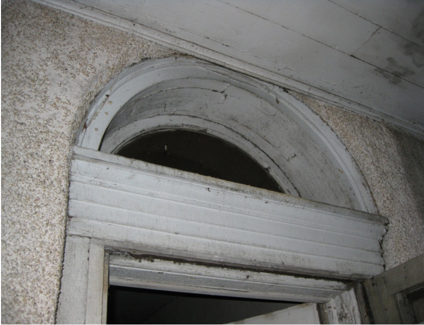
Image of front door exterior with fan light from October 2009: note truncated trim at top of window
