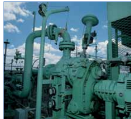
A pressure letdown installation recovers 1,000,000 kWh/yr from a southern California, US municipal natural gas pipeline.
