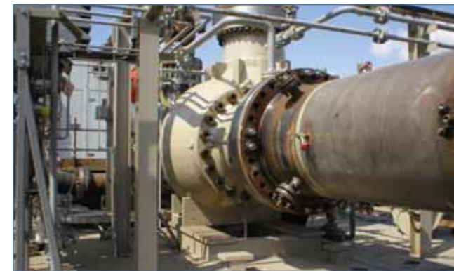
A GE turboexpander test facility.
