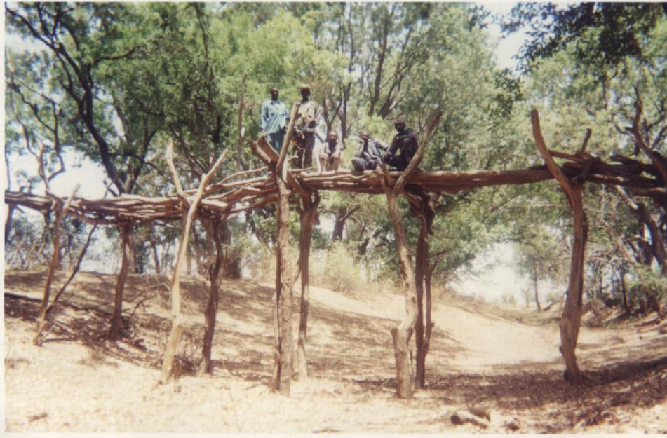
Plate 15. A wooden bridge made to access the protected area during the flood season.
