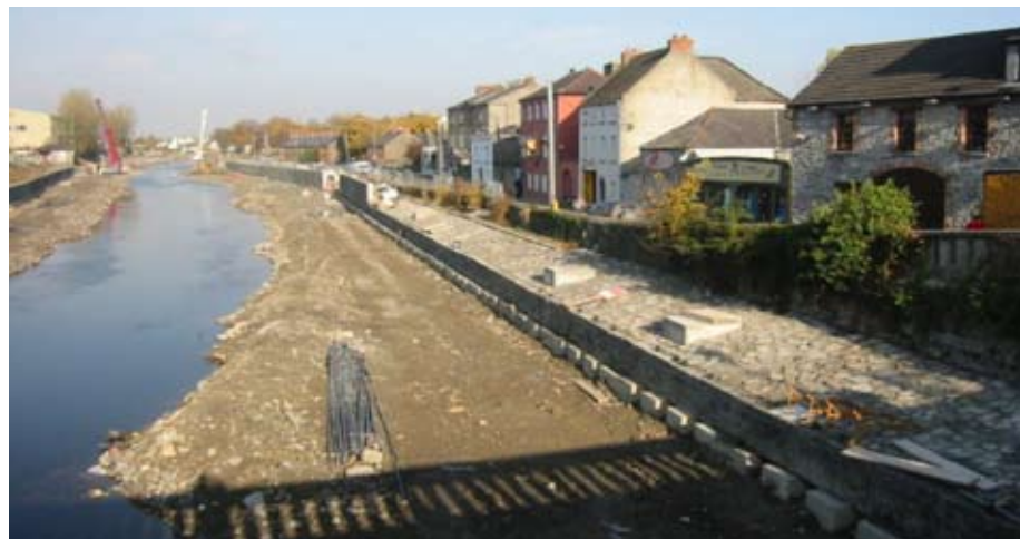
Construction of new masonry wall as part of OPW flood relief scheme in Kilkenny
