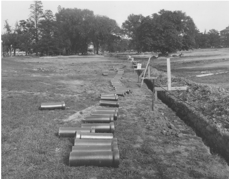
Grading and the laying of utilities on the Mall. In the distance can be seen some of the tree wells built around mature trees to be moved. (from MRCE; CLP file "Mall grading 7-12 Sts")
