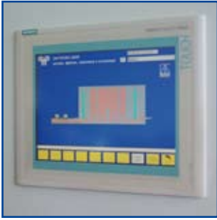
The control display of the final proofer. All parameters can be adjusted and recalled in a functional and clearly arranged manner.
