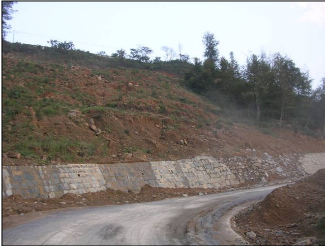
Figure 17-12: Unstable Slope on Main Access Road to Plant, 15 October 2006
