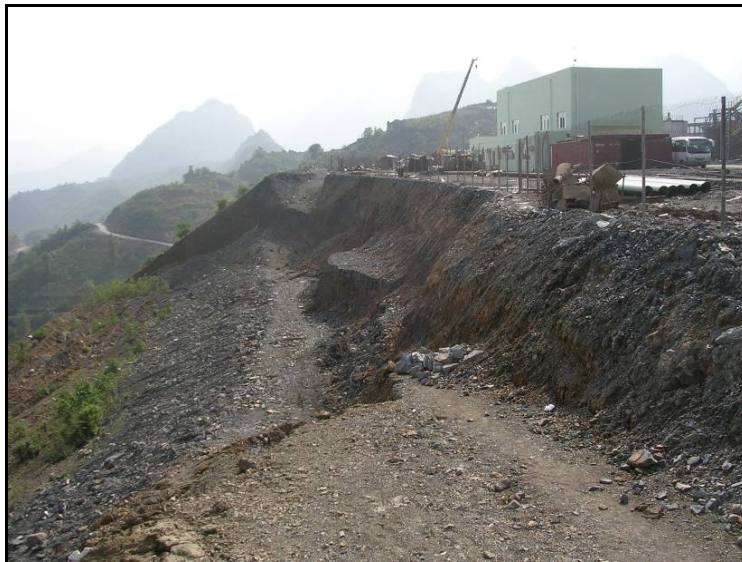
Figure 17-26: Photograph Showing Plant Site Embankment Failure, 15 October 2006
