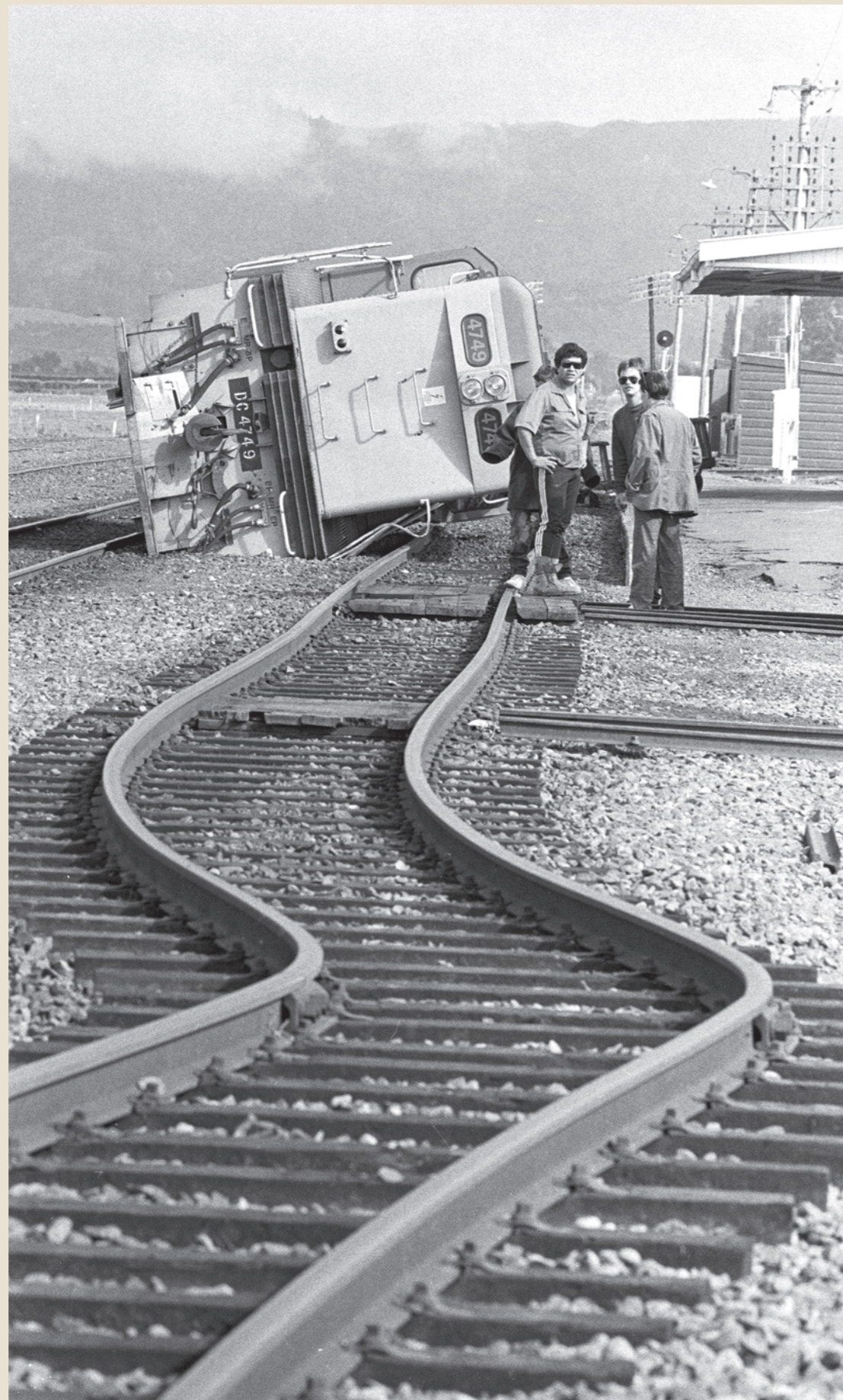
In the Edgecumbe rail yards, an 80-tonne locomotive lies on its side. The heavier main shock caused the tracks to buckle, toppling the locomotive.
